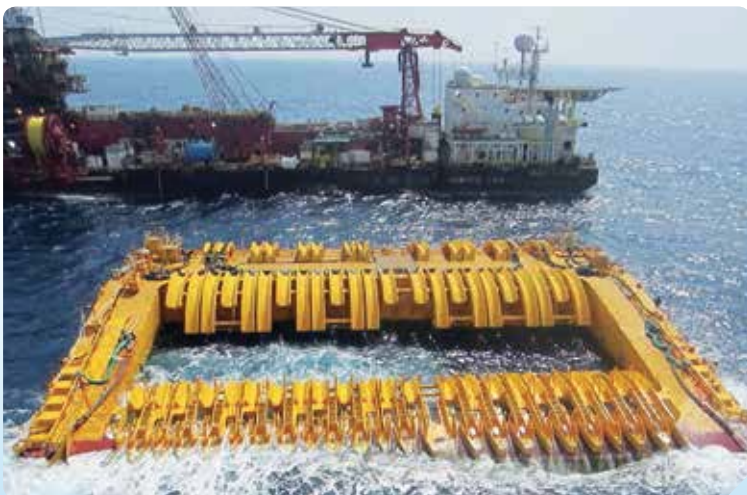
One of the four Buoy-Supported Risers (BSRs) now installed and operational on the Guar-Lula NE SURF project in Brazil
